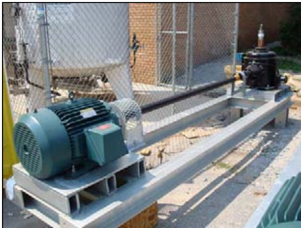
Figure 1: Typical Fan Drive Arrangement
