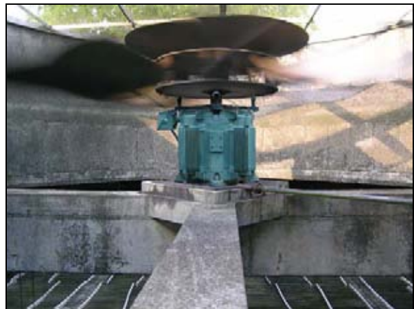
Figure 7 – PM Motor Installed in Place of Gearbox & Driveshaft
