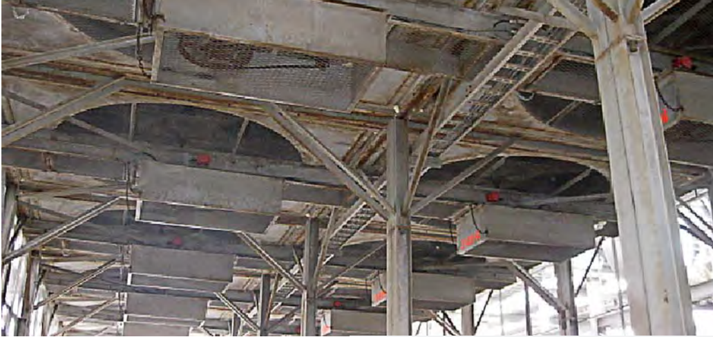
Above: Typical bottom view of a gas plant cooling bank
