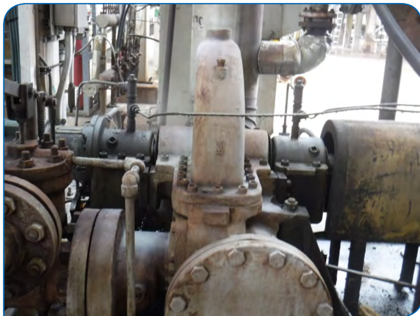
Outdoor boiler feed pump at a refinery in Canada with thermal growth issues due to seasonal pipe strain.
